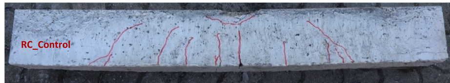
Fig. 14. Condition of RC_Control at the end of the test.
