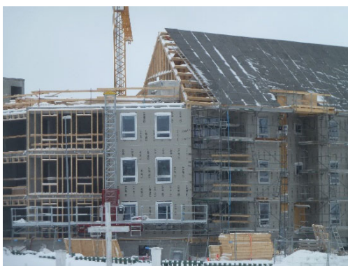
Figure 3. Multi-storey building with wood-based facades before and after installing wind barrier, and wood-based roof construction with roofing felt.
