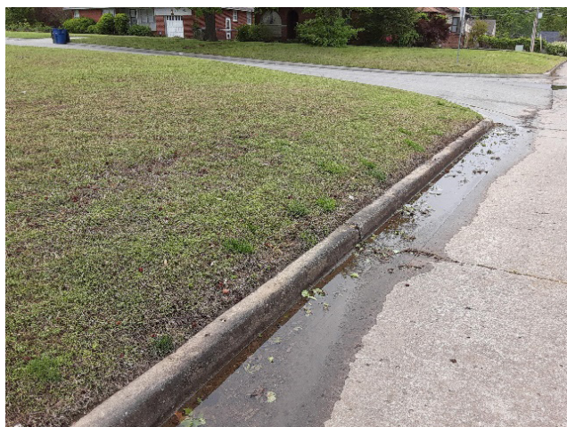
Figure 5. Seepage faces exist at many areas, where the water table reaches the surface. Water in a road with no other source (irrigation, etc.) detected and a wet soil surface near the curb.
