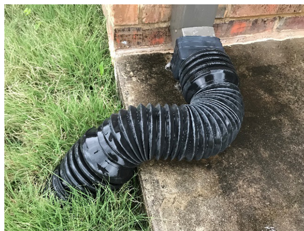
Figure 3. Connecting downspouts with drains can help in routing water away from the foundation of the house to a location better suited to handle the large volume of water deposited on-site during heavy rainfall.
