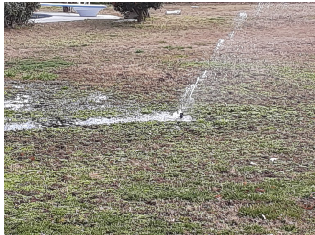
Figure 4. Waste treatment system impact-type sprinkler for distribution of treated waste. The dog has also broken the sprinkler head, causing added water problems.
