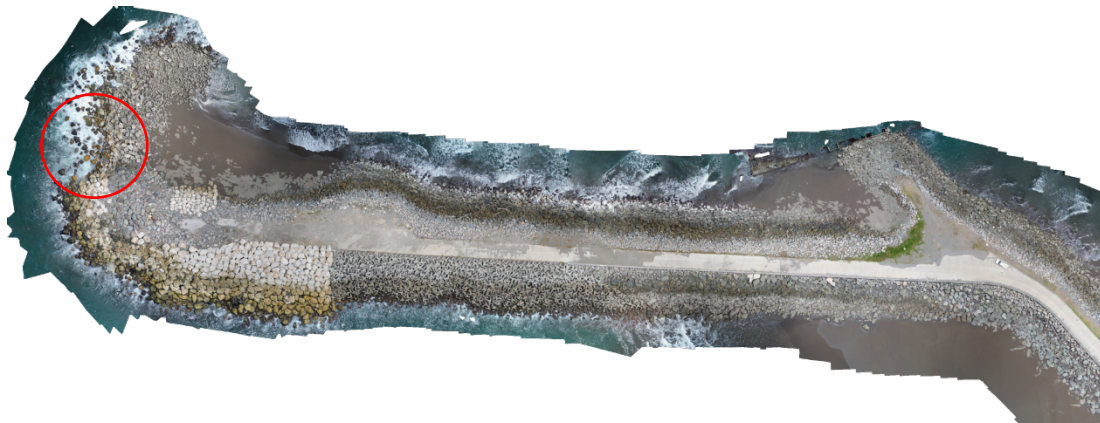
Figure 5. Caldera Port Breakwater heads damage.
