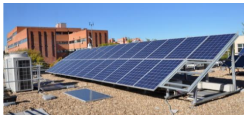
Figure 1: PV Array 1, with a peak power of 5.8 kWp.
