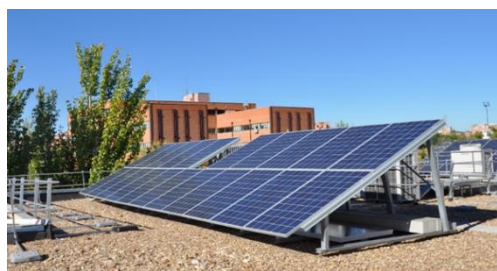
Figure 2: PV Array 2 with a peak power of 5.1 kWp.
