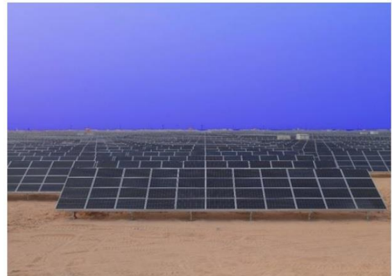
Figure 1. Adrar's PV power plant
