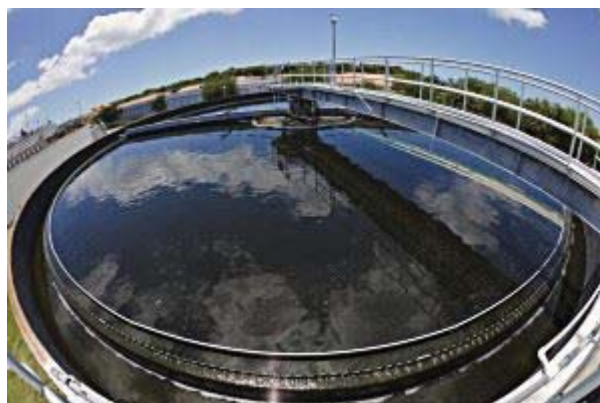
Figure 9. Secondary clarifier of the secondary stage treatment [39a]
