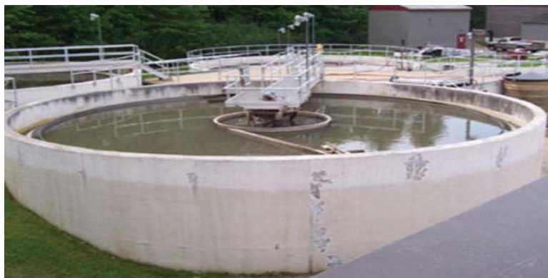
Figure 7. Circular primary clarifier tank of a wastewater treatment plant [36a]
