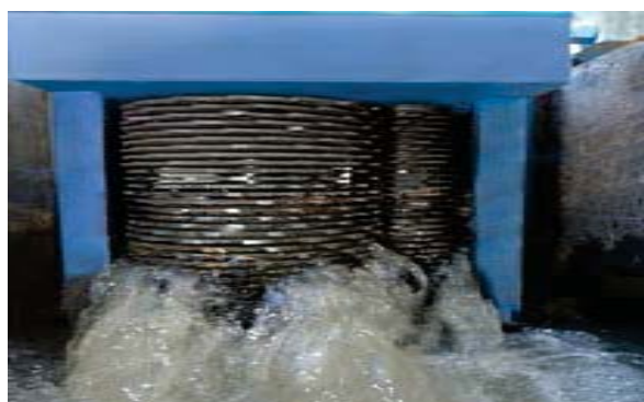
Figure 5. Comminutors of wastewater [31a]
