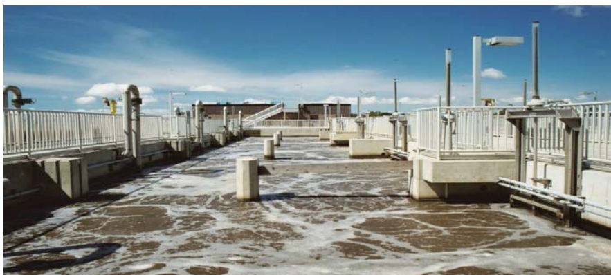
Figure 8. Aeration tank of the secondary stage treatment [39a]
