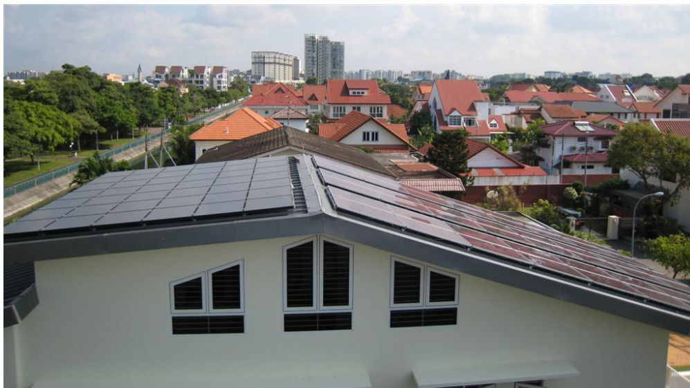
Figure 6.1: The first zero energy house in Singapore. Rooftop panels on the right and left have inclination of 18.3^\circ and 6.1^\circ ; azimuth rotation (north is 0^\circ ) 66^\circ NE and 246^\circ SW respectively.
