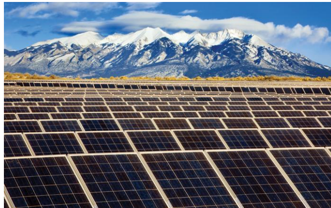
Figure 6.6: Photograph of a typical PV system.
