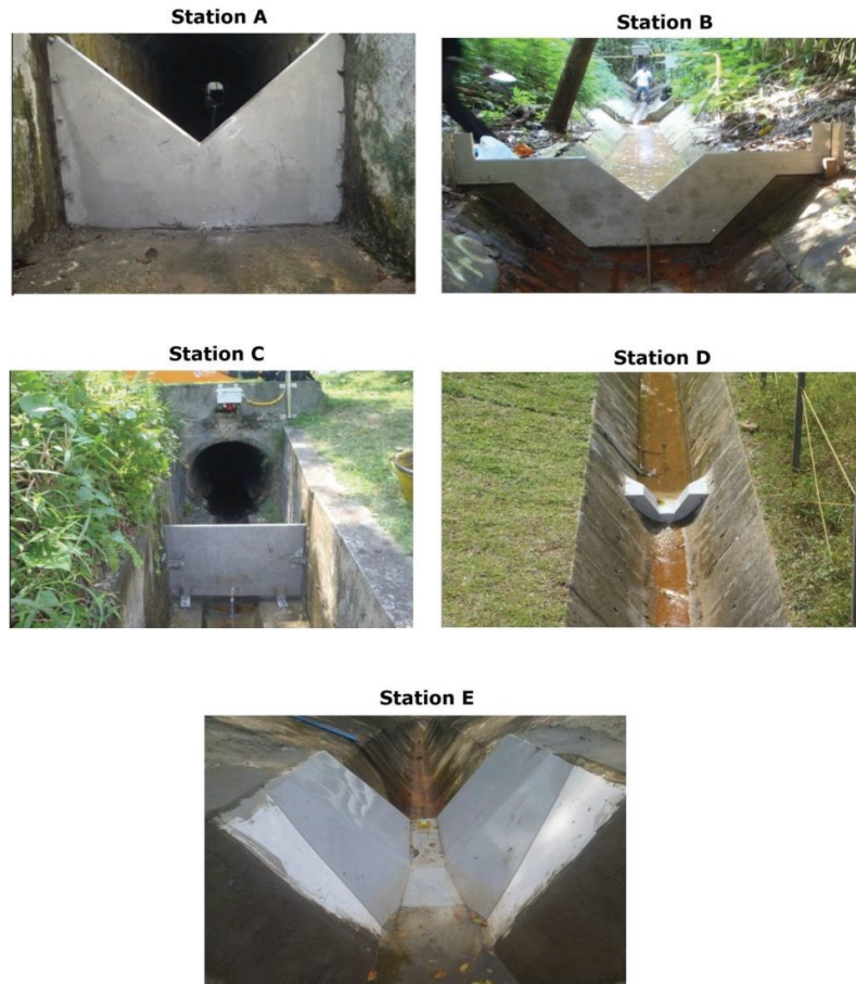
Figure 3.4: Types of control structure for streamflow monitoring stations within Kent Ridge Catchment, Singapore
