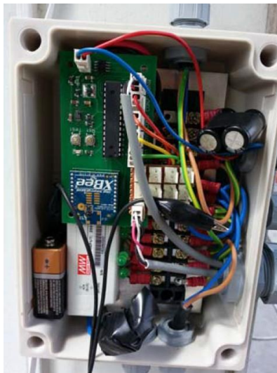
(a) Central control station
