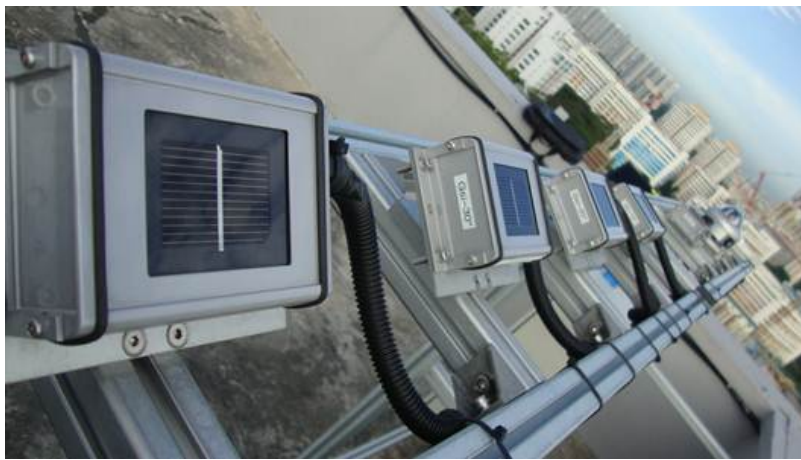
Fig. 7.2 Photograph of the irradiance measurement station located on the rooftop of Solar Energy Research Institute of Singapore (SERIS).
