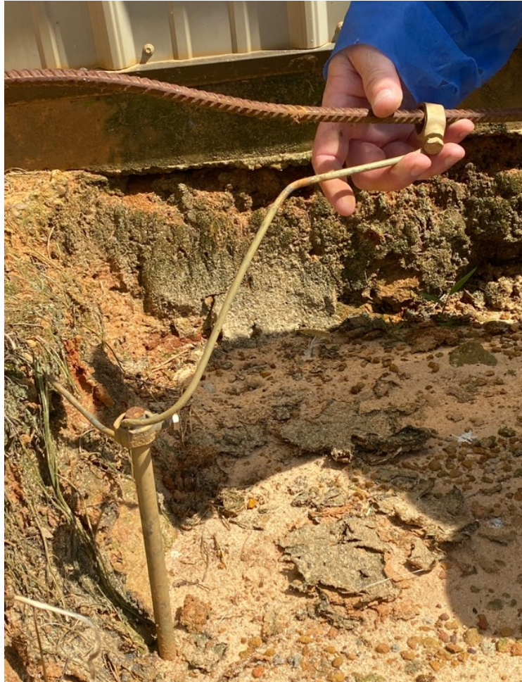
Figure 2.4 Disconnected ground on surveyed broiler farm.
