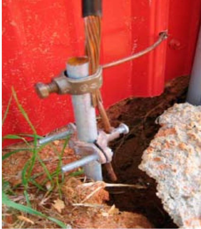
Figure 2.1 Proper electrical ground outside a broiler production facility utilizing acorn clamps.
