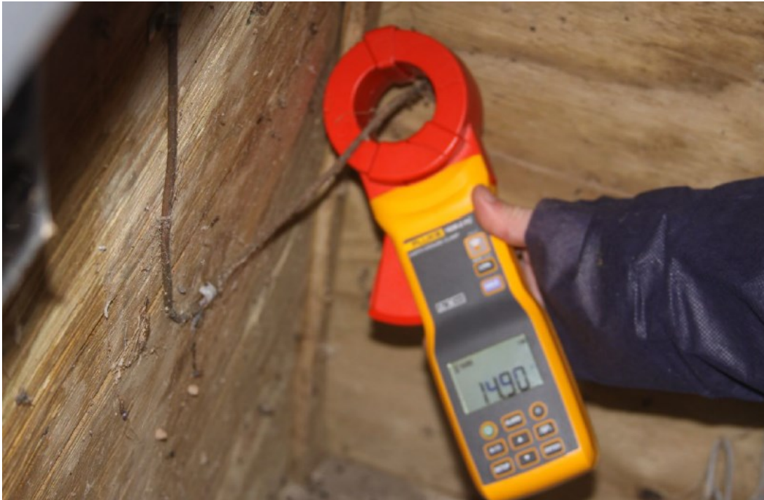
Figure 2.3 Fluke earth resistance meter used to collect grounding resistances.
