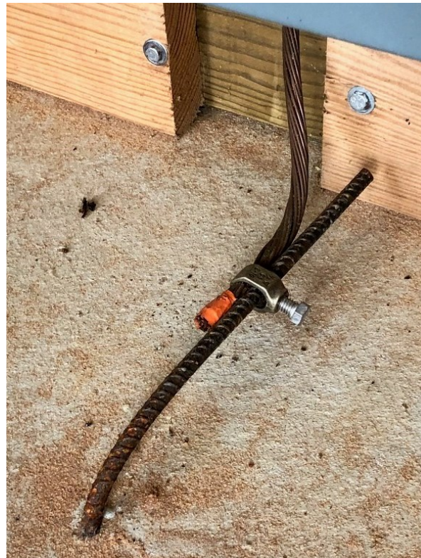
Figure 2.2 Ufer grounding connection on the generator service panel of a broiler farm.
