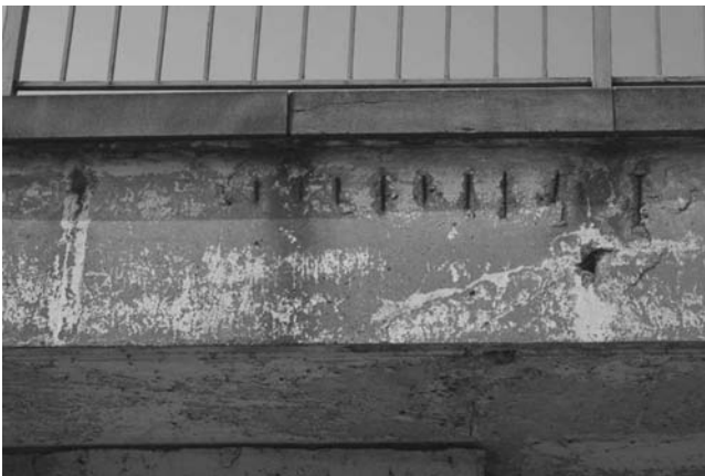
Figure 3.6 Reinforcement corrosion in case of insufficient cover thickness.
