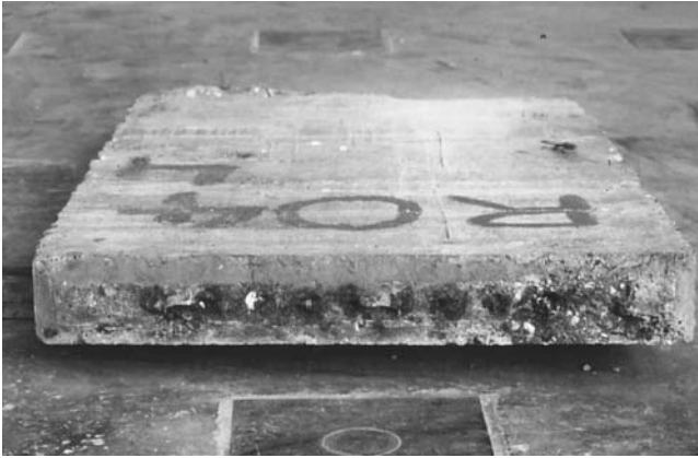
Figure 2.4 View of failed hinge of tensile pendulum pillar (with corroded prestressing wires).
