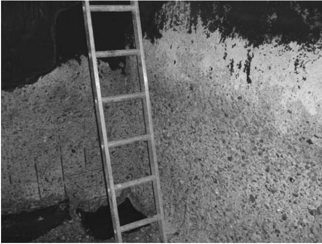
Figure 5.34 Sulfuric acid attack on a concrete wastewater tank in an industrial plant (courtesy of SCICON Worldwide bvba).
