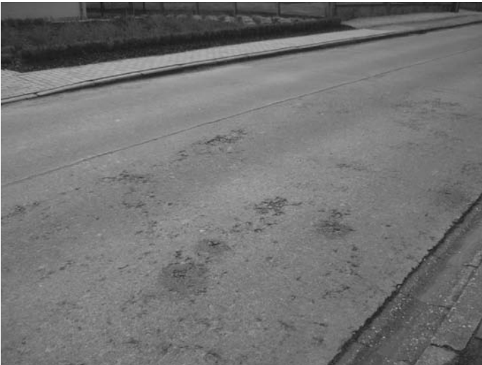
Figure 5.12 Salt scaling on a concrete road.
