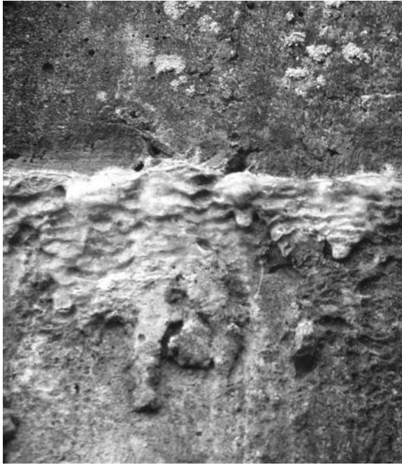
Figure 5.21 Formation of calcium deposits.
