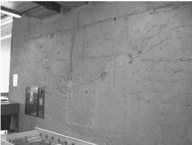
Figure 3.8 Visual defects due to inappropriate compaction of a concrete wall.
