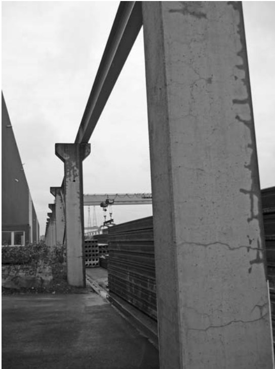
Figure 5.27 ASR in concrete columns.
