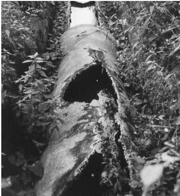
Figure 5.35 Biogenic sulfuric acid attack in a concrete sewer system, totally damaging the upper part of the concrete pipe above the wastewater line.
