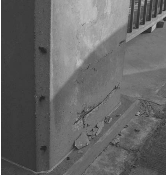
Figure 5.45 Carbonation-induced corrosion in a column.
