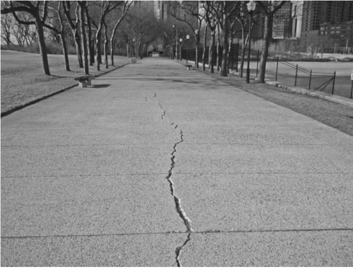
Figure 4.5 Drying shrinkage cracking in walkway.
