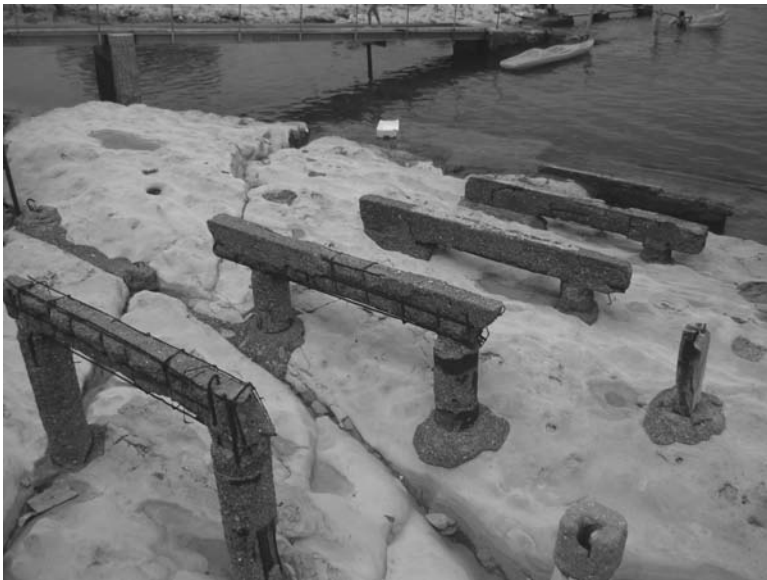
Figure 5.47 Chloride induced reinforcement corrosion in some concrete elements near the Adriatic Sea.
