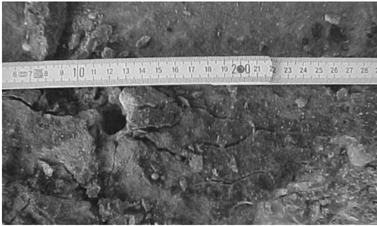
Figure 5.30 Detail of a concrete balcony damaged by expansive chemical sulfate attack (courtesy of SCICON Worldwide bvba).
