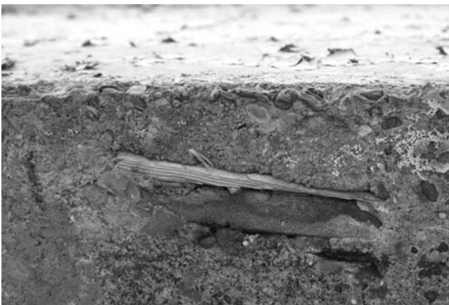
Figure 3.10 Unwanted inclusions in concrete.
