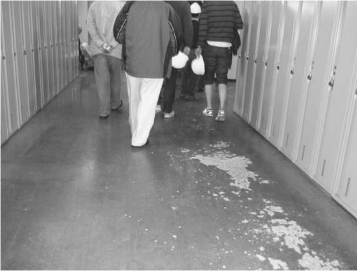
Figure 5.13 Abrasion of concrete floor by intensive walking and sliding near a range of lockers.
