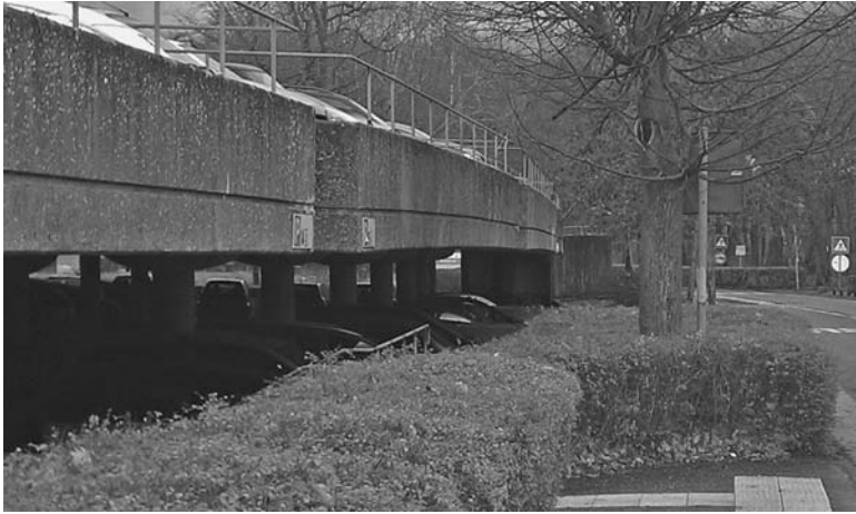
Figure 2.8 Long-term creep deformations of concrete parking structure.
