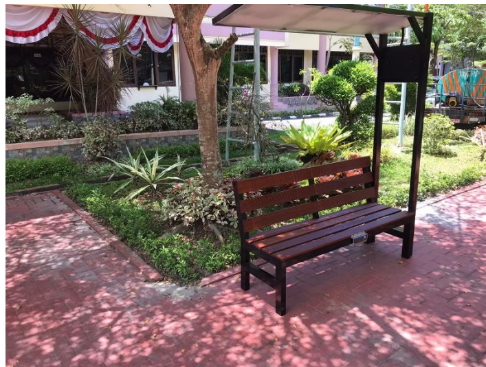
Figure 8. Implementation of benches with solar panels in the garden area
