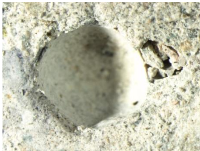
Fig. 4. C-32-Bottom-1: Voids filled with crystalline material
