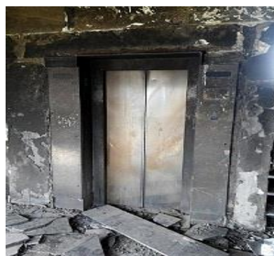
Fig. 2. View of lift lobby in fire damaged area
