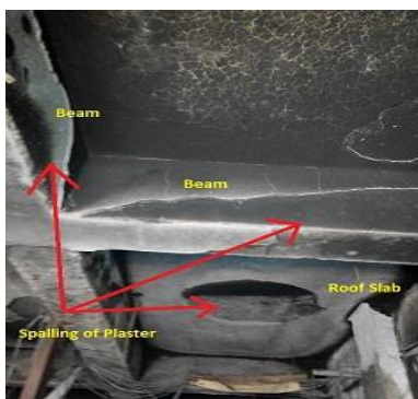
Fig. 1. Spalling of Plaster in Beams & Slabs
