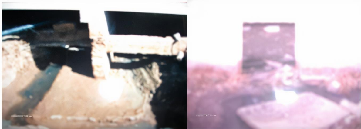
Fig. 3. The soil of foundations is completely saturated and sanitary collector were damaged.
