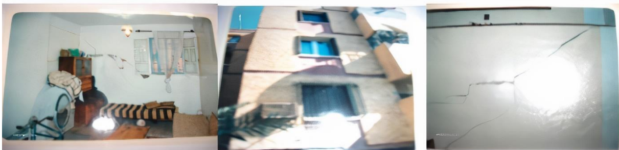
Fig. 2. Cracks in exterior and interior walls
