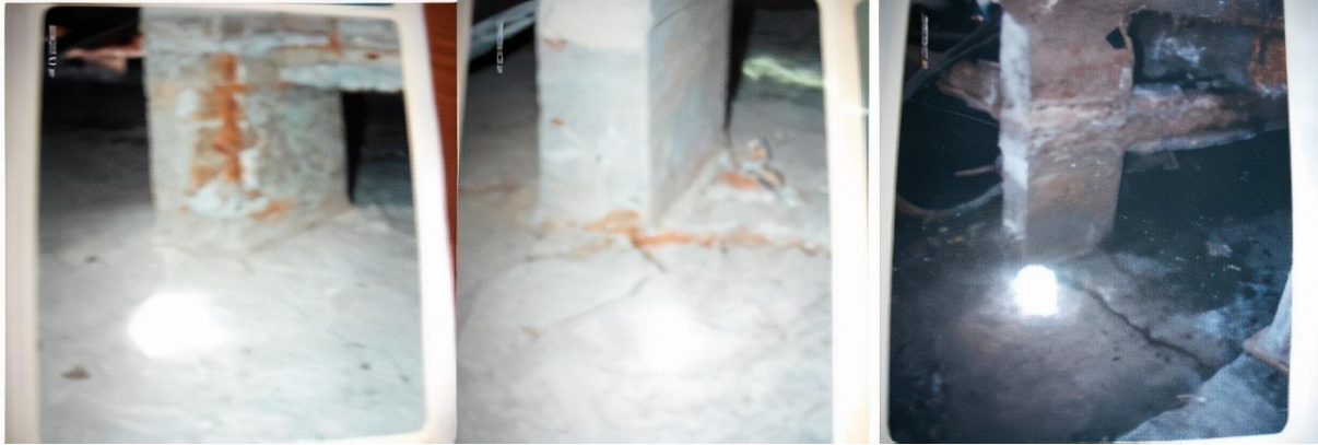
Fig. 4. Primary columns rusted and important cracks in foundation.
