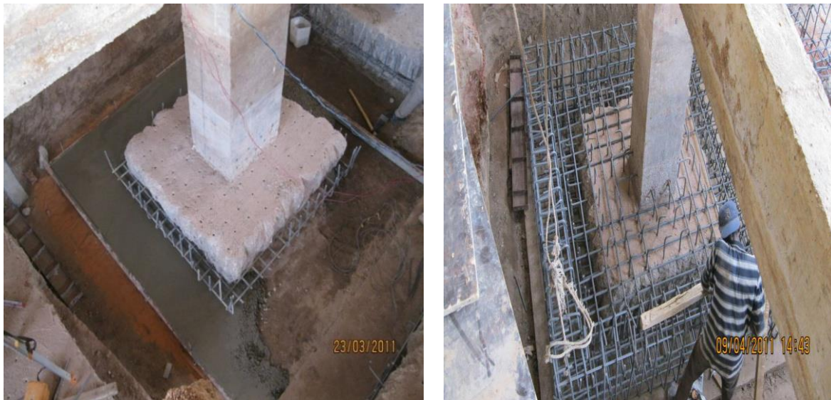
Fig 6. Plain concrete in the extended area and the reinforcement bars arranged surrounding the footing.
