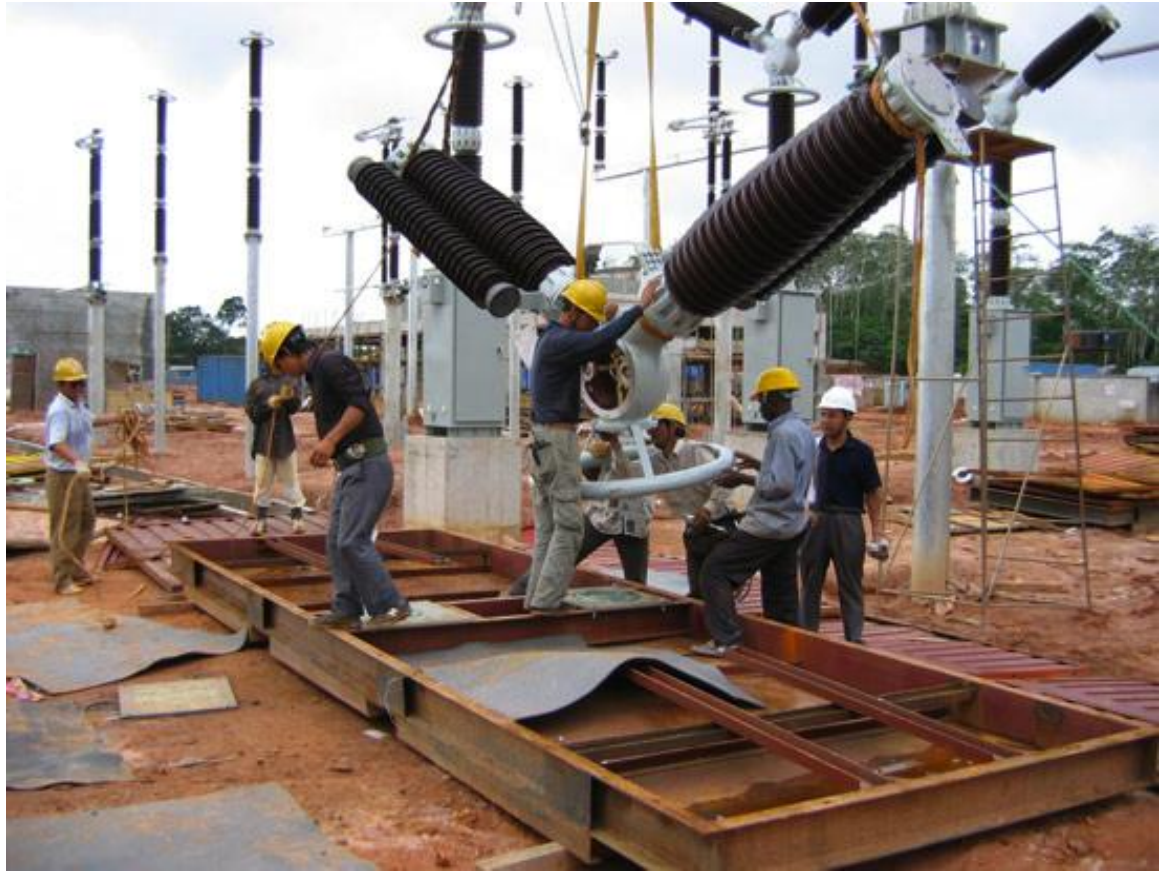
Figure 8.12: Case Study 4 project site (during an earlier stage of phase 2 of the project)
