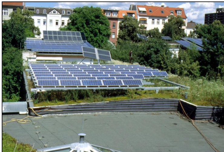
Figure 2.16. PV arrays on green roof in Germany Source: Kohler (2002)
