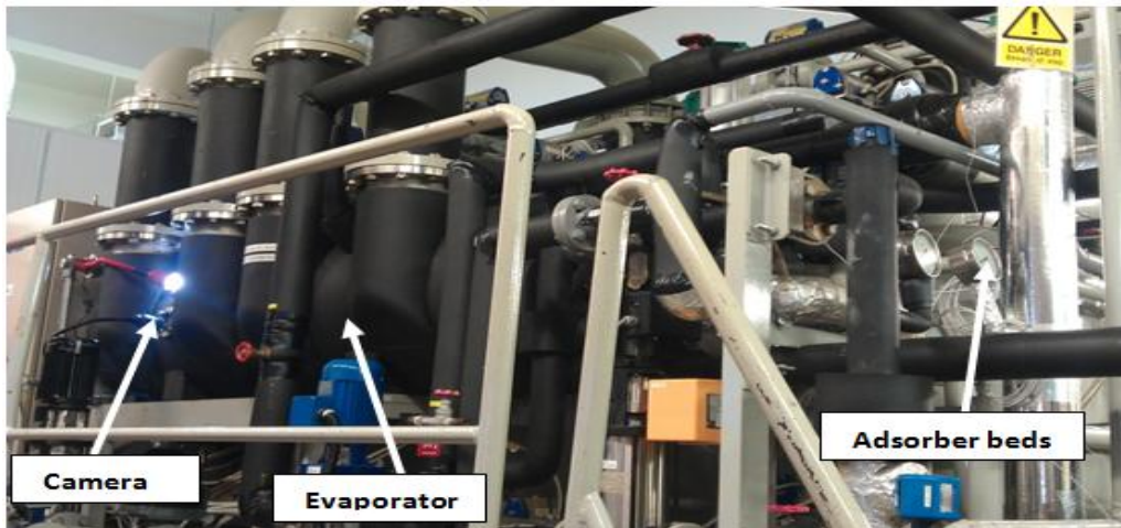
Figure 3.1 Pictorial view of adsorption desalination plant installed in NUS
