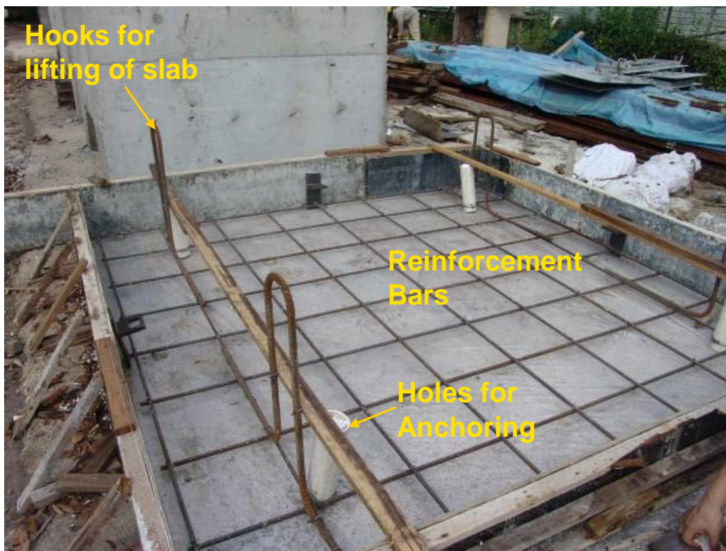
Figure 4.4 Minimal reinforcement at bottom of slab
