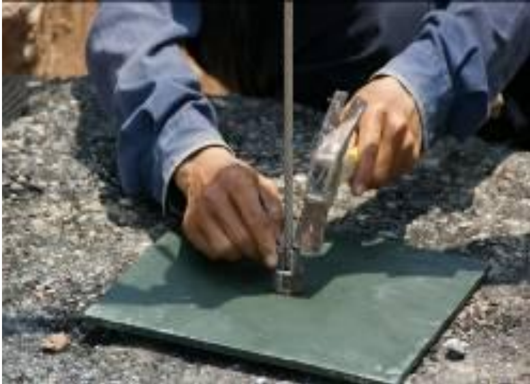
Figure 4.10 Extraction of steel cable using excavator & anchoring of steel plates on surface of slab
