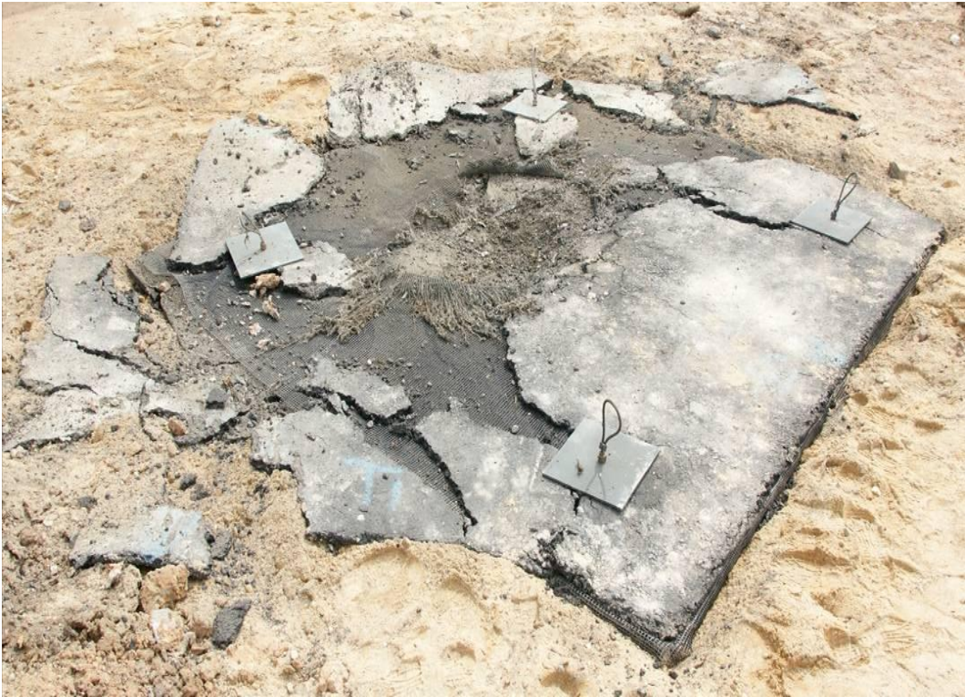
Figure 6.41 Damage of proposed multi-layers pavement after blast
