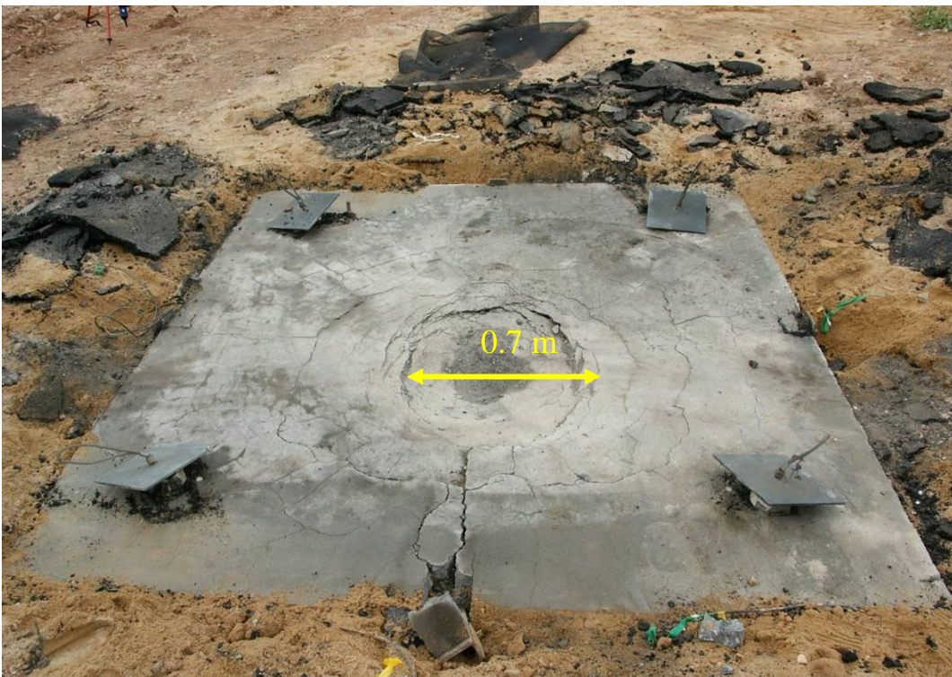
Figure 6.42 Damage of proposed multi-layers pavement after blast (Removing asphalt layer)
