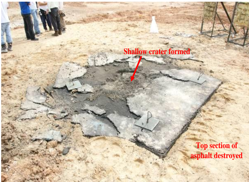
Figure 4.35 Slab 2 after blast
