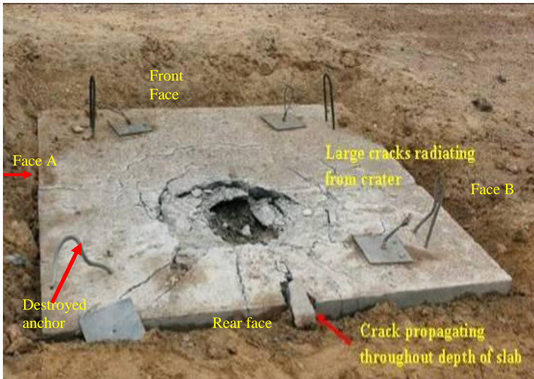
Figure 4.22 Slab 1 after blast
