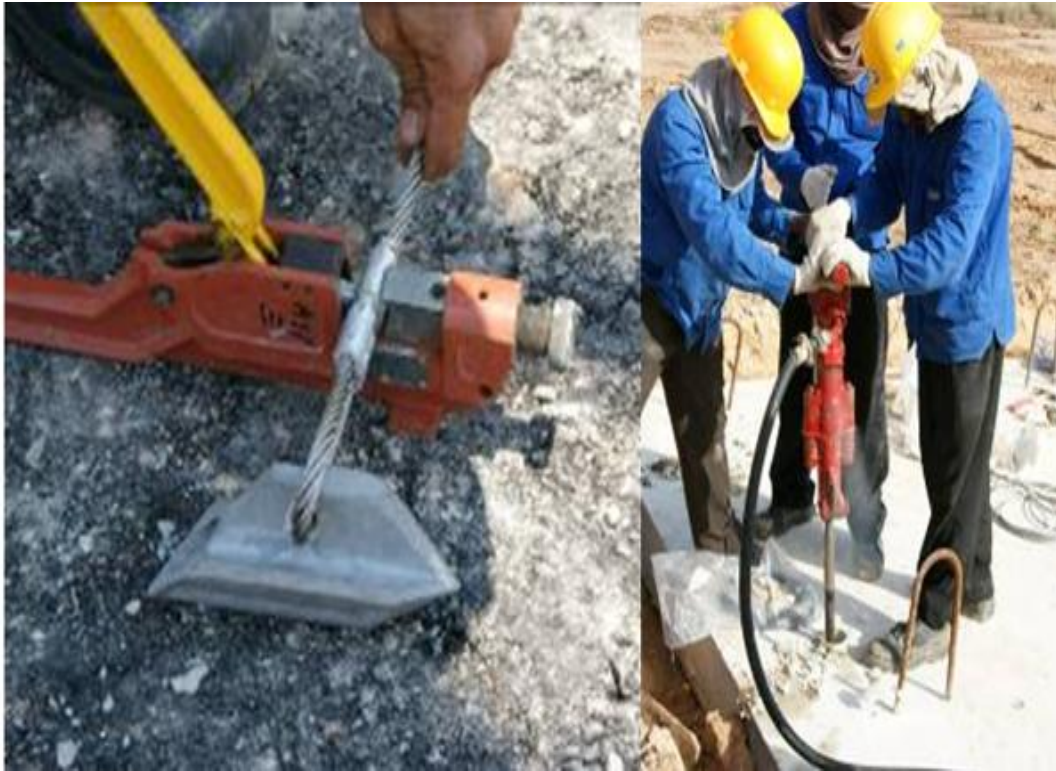
Figure 4.9 Attachment of steel cable to anchor & driving in of the anchor using an air compressor
