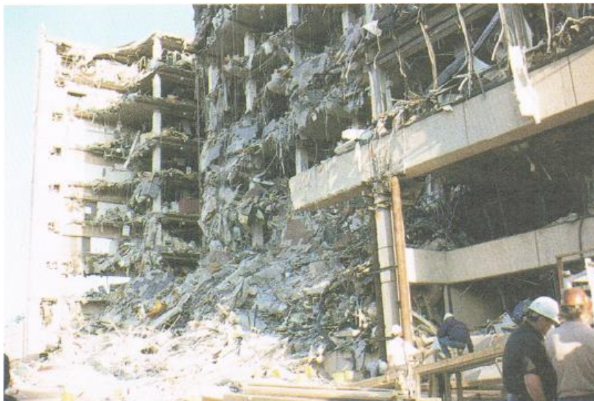
Figure 1.3: Partial collapse of Alfred P. Murrah Building (Hinman and Hammond, 1997)
