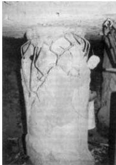
Figure 1-6 Pile damaged due to excessive bending moment induced by superstructure inertial forces during the 1995 Kobe Earthquake (Tokimatsu et al. , 1996)
