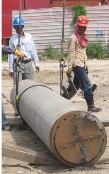
Figure 5-22 The steel cap welded to the pile toe to form the closed-ended pile.
