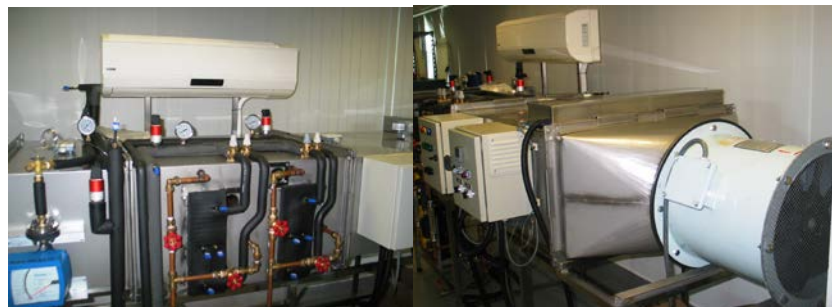
Figure 5.2 Photograph of the evaporatively cooled condenser split air-conditioner
