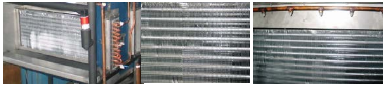
Figure 5.3 Photograph of the finned evaporatively-cooled condenser
