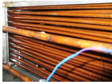
Figure 5.4 Photograph of the finned evaporatively-cooled condenser
