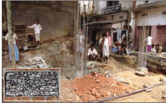
Figure 77: The demolished Churihatta mosque site showing the construction of the new block, source: Ghias, 2008b, July 28.
