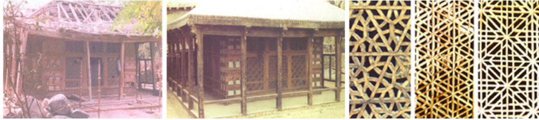
Figure 14: Astana of Syed Mir Muhammad before and after stabilization and restoration, right: Delicate geometry of the wooden lattice screens, source: UNESCO, 2007, pp. 267-268.
