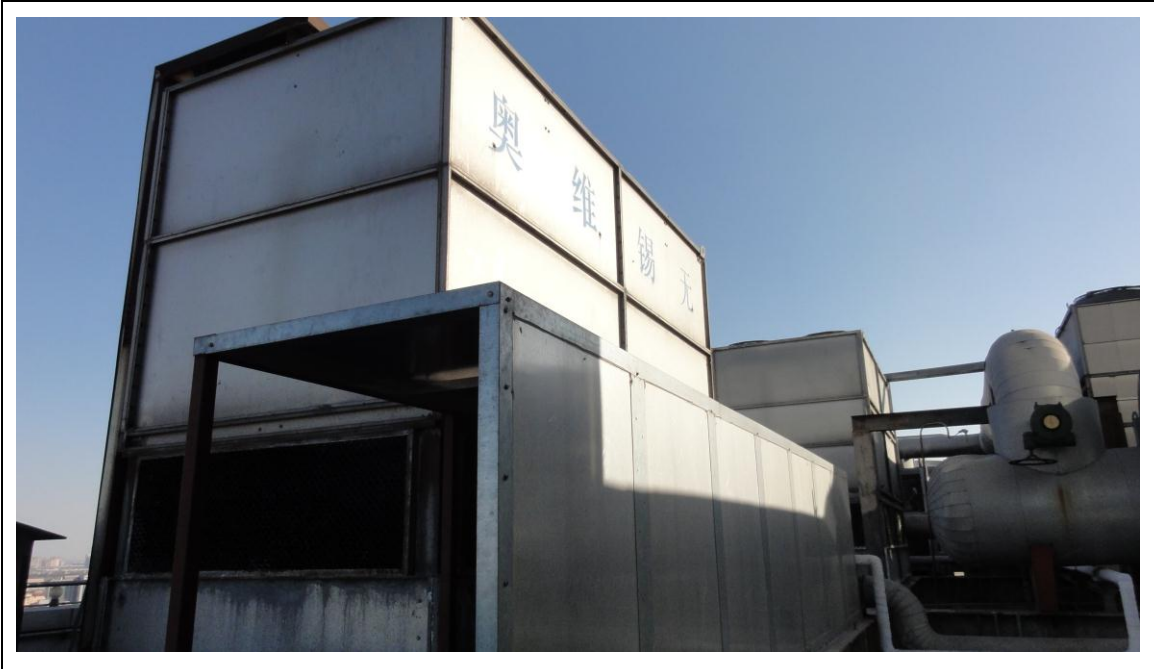
Figure 19: Intelligence Green Cooling System Installed at Roof Top of China Mobile's Beijing Subsidiary Office
