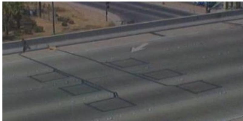
Figure 4.3 Induction loop detectors at intersection
