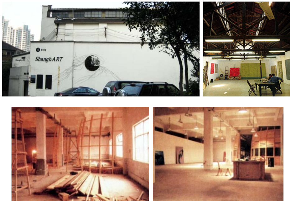
Figure 141 Pictures of exterior and interior renovations in Chunming Textile Factory in the 2000s.
