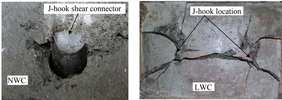
(a) Shearing failure of connector
