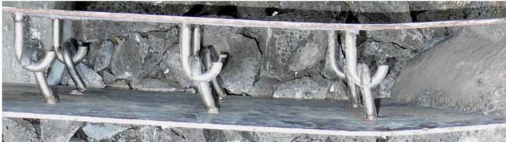
(c) Shear connector failure
