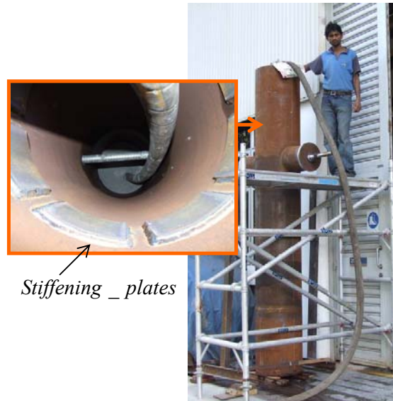
Figure 3.9 Grouting the specimen: keeping the trimie hose out-let below the grout surface
