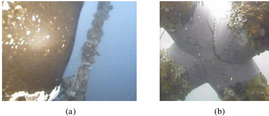
Figure 1.1 Typical failures of components of existing jacket structure: (a) local buckling of leg member, (b) cracking and fracture of X joint. Extracted from Energo Engineering (2007)
