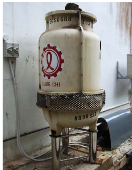
Figure 9.15 Cooling tower and external pump
