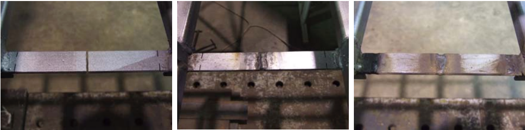
Figure 6.7: Progressive strengthening at one level by welding: strengthening baseline (left), moderate strengthening (middle), large strengthening (right)
