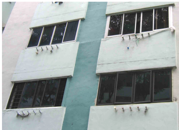
Figure 3. 8 Cloth drying facilities on the external wall of kitchen of Building One
