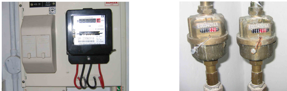
Figure 3. 5 Electricity meter and water meters outside residential units
