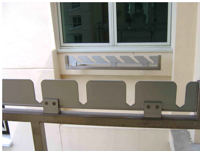
Figure 3. 14 Cloth drying facilities on the external walls of bedroom and kitchen in Building Two
