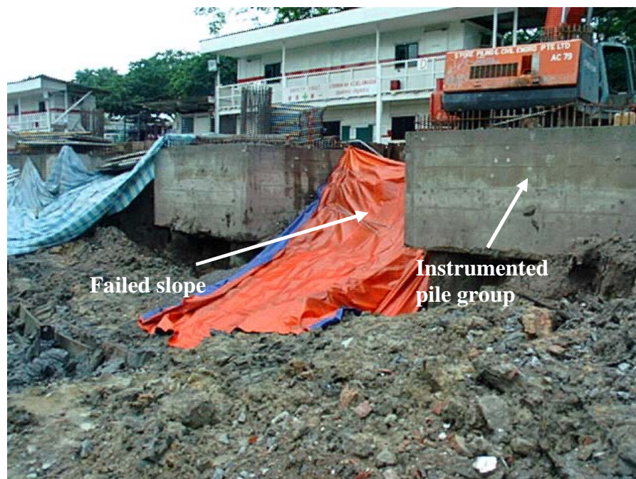
(b) Slope failure next to instrumented pile group (12 Dec 2002)
