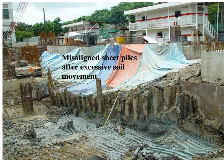
(f) Another view of deflected sheet piles due to excessive soil movement (26 Dec 2002)
