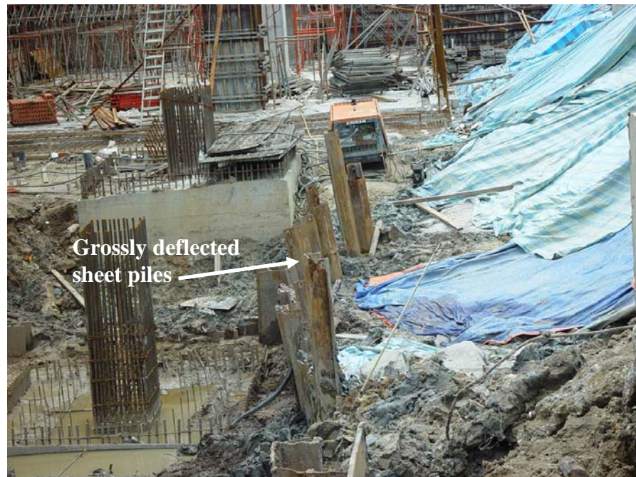
(e) Deflected sheet piles due to excessive soil movement (26 Dec 2002)
