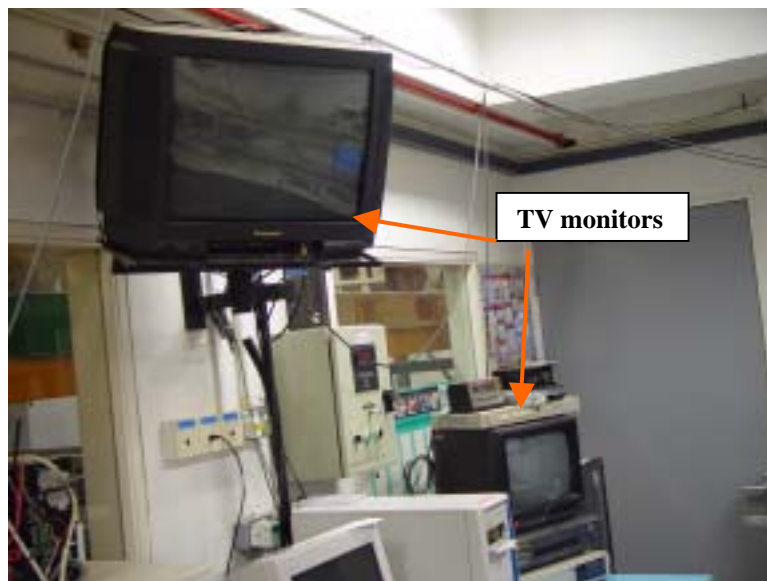
Figure 3.4 TV monitors in control room
