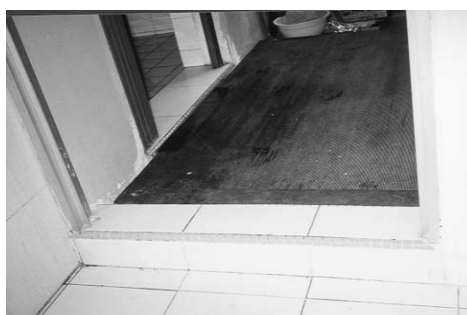
Figure A4.1: Thresholds between kitchen and bathroom made the bathroom inaccessible.
