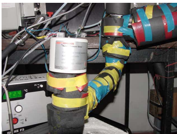
Figure 4.2 (b) Flexible hose between evaporator and reaction tube
