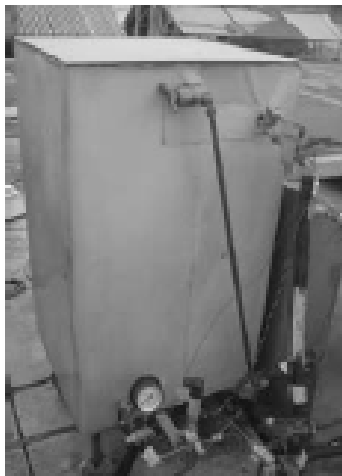
Figure 3.6. Water condenser tank
