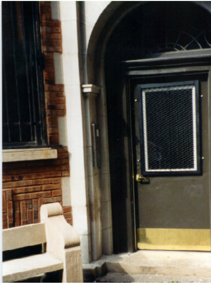
Figure 25. One of the upgraded doors funded by the SECURE project.
