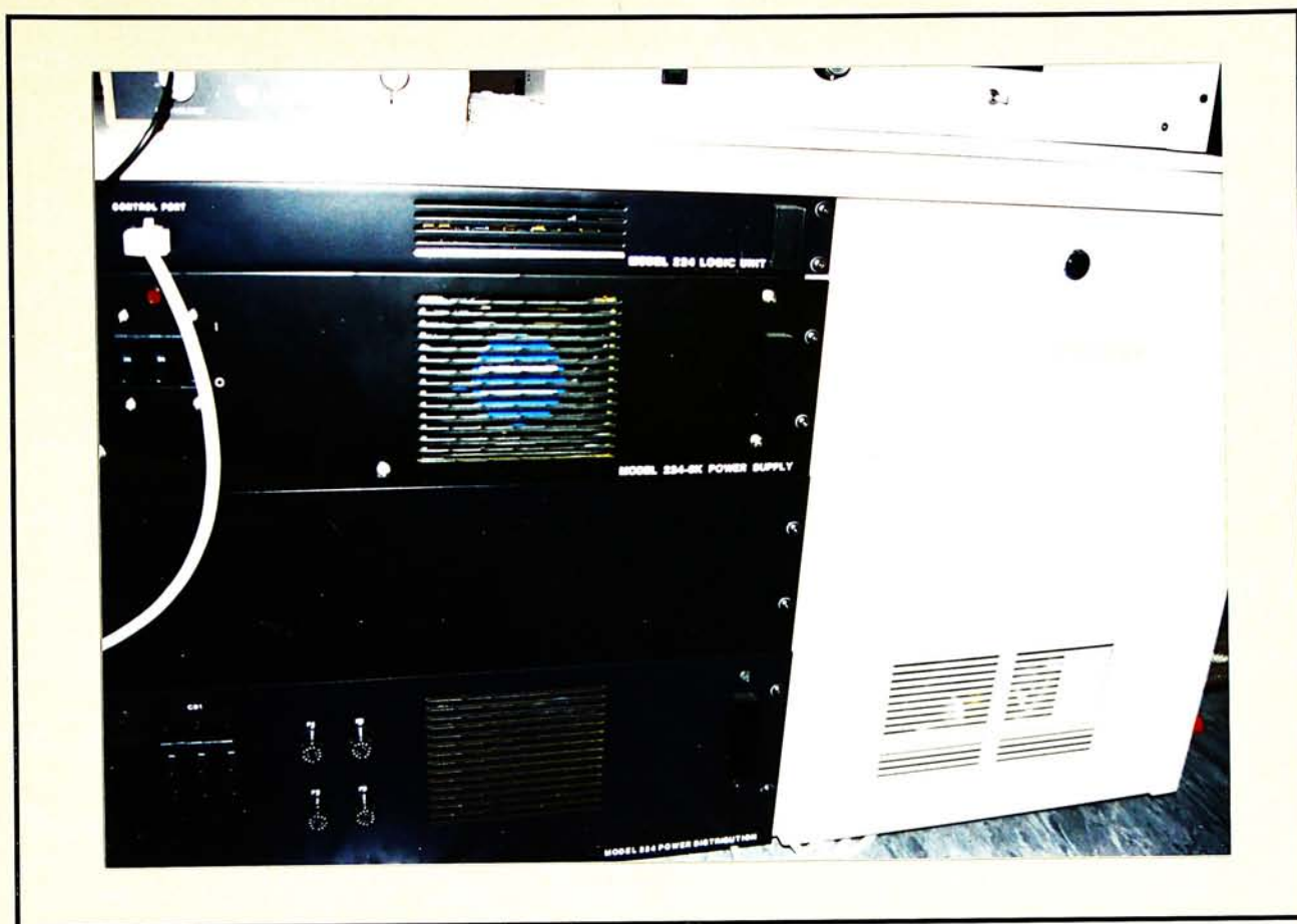
Figure A1-pIV The logic control unit, in which a power control unit and a primary cooling system are installed.
