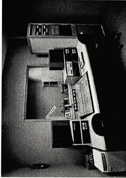
Control Room of Audio Studio
