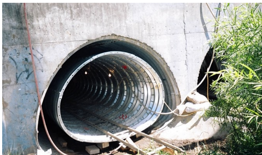
FIGURE 1.21 The liner, the pipe and space to be filled (grouted). (Source: theconstructor.org. )
