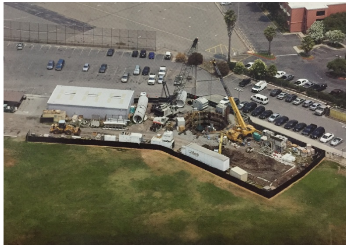
FIGURE 1.59 Let the project begin: the project used an earth pressure balance machine to install a 2.400 mm ID RCP. (Source: ISTT. )
