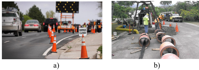
FIGURE 1.55 Potential risks. a) Proper signals and barriers b) Limited barriers without signal. (Source: ISTT. )
