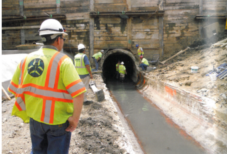
FIGURE 1.20 Installation of 2.250 mm diameter fiberglass pipe into an existing utility sewer. (Source: ISTT, 2014 )
