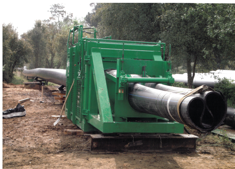
FIGURE 2.10 Pre-welded polyethylene pipe sent through a former into “hearth shape” in preparation for installation into host pipe. (Source: ISTT)
