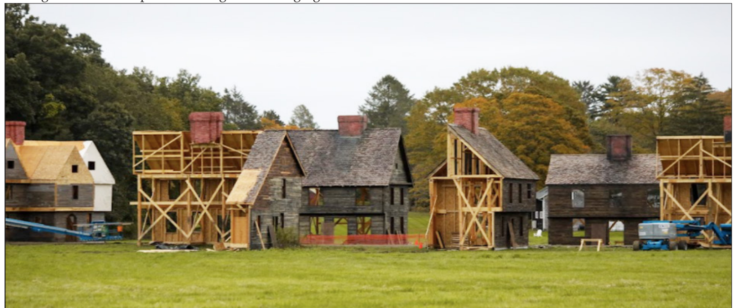
A set in Lincoln, RI being constructed for the filming of Hocus Pocus 2 .
