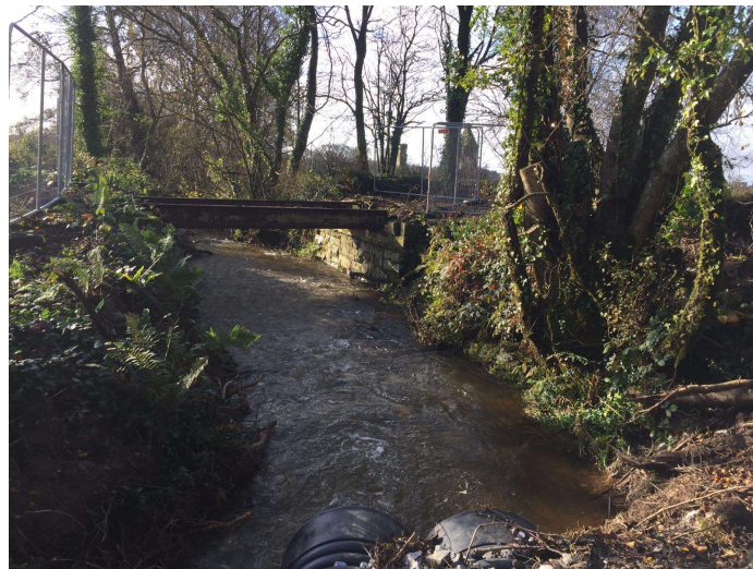
Figure 3. Existing structure on greenway route at Roxborough, showing steel girders and masonry abutments
