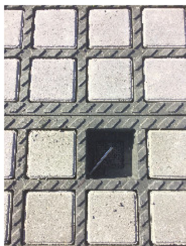
Figure 4. Example of sensor position at a depth of 3 cm in concrete paving stones (CS107). The sensor was placed inside a paving stone.
