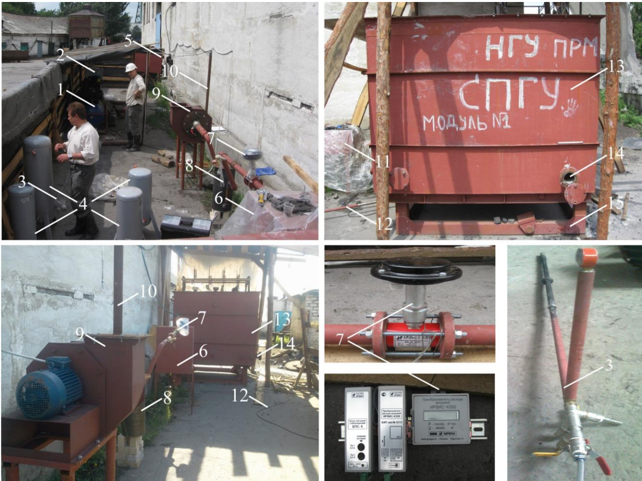
Fig. 1. General view of the operating systems: 1 – compressor RM-3138; 2 – steam generator AVPE-11/9; 3 – high-pressure pipeline; 4 – receiver (air, steam and oxygen); 5 – a water reservoir; 6 – a tank-cooler; 7 – flowmeter IRVIS-300C; 8 – lime filter (catching of H_2S ); 9 – exhauster DR-1,0-00.00PS; 10 – offtake; 11 – tank of dew and slags collection; 12 – flexible pipeline; 13 – the stand setting; 14 – ignition borehole; 15 – platform for coal seam angle simulation
