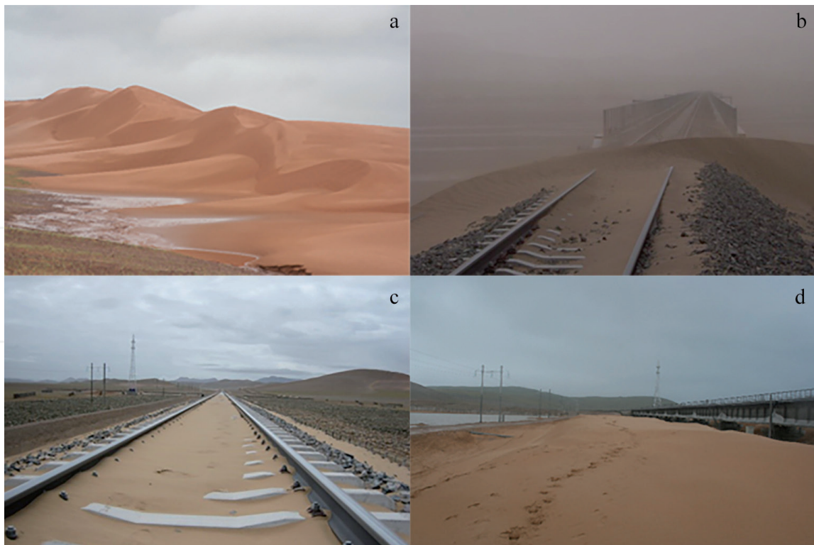
Figure 1. Sand disasters along the Qinghai-Tibet Railway. (a) Hongliang River section, (b) Tuotuo River section, (c) Za'gya Zangbo section, (d) Cuona Lake section.
