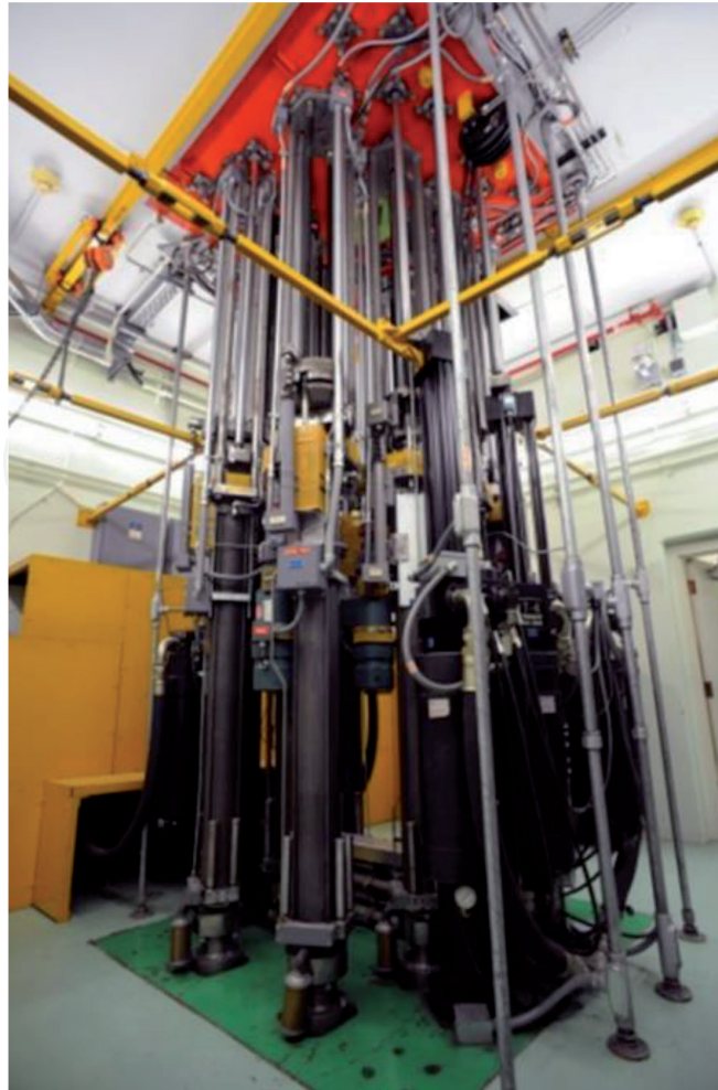
Figure 6. View of TREAT rod drive mechanisms from the sub-pile room.
